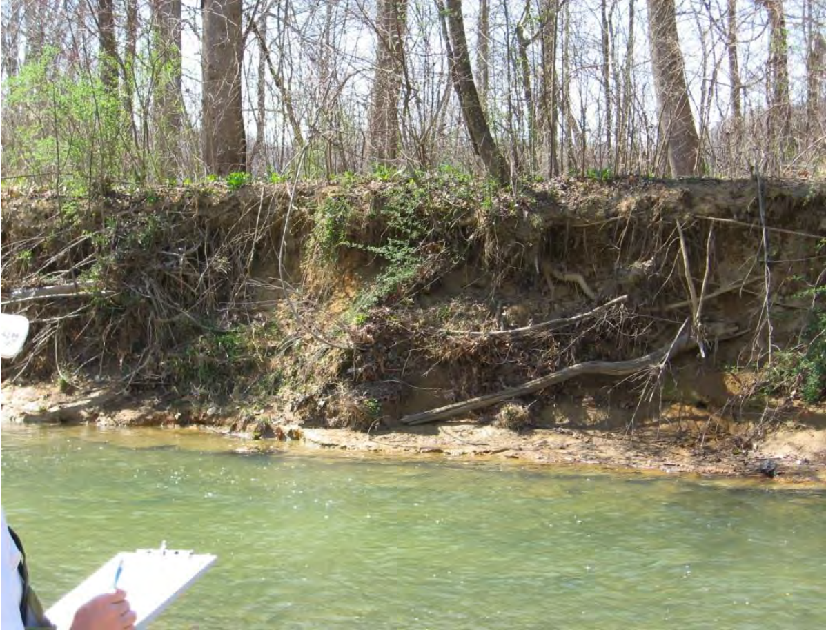
Figure 3.52. Example of a streambank with high erosion risk (MBEHI = 21.8).
