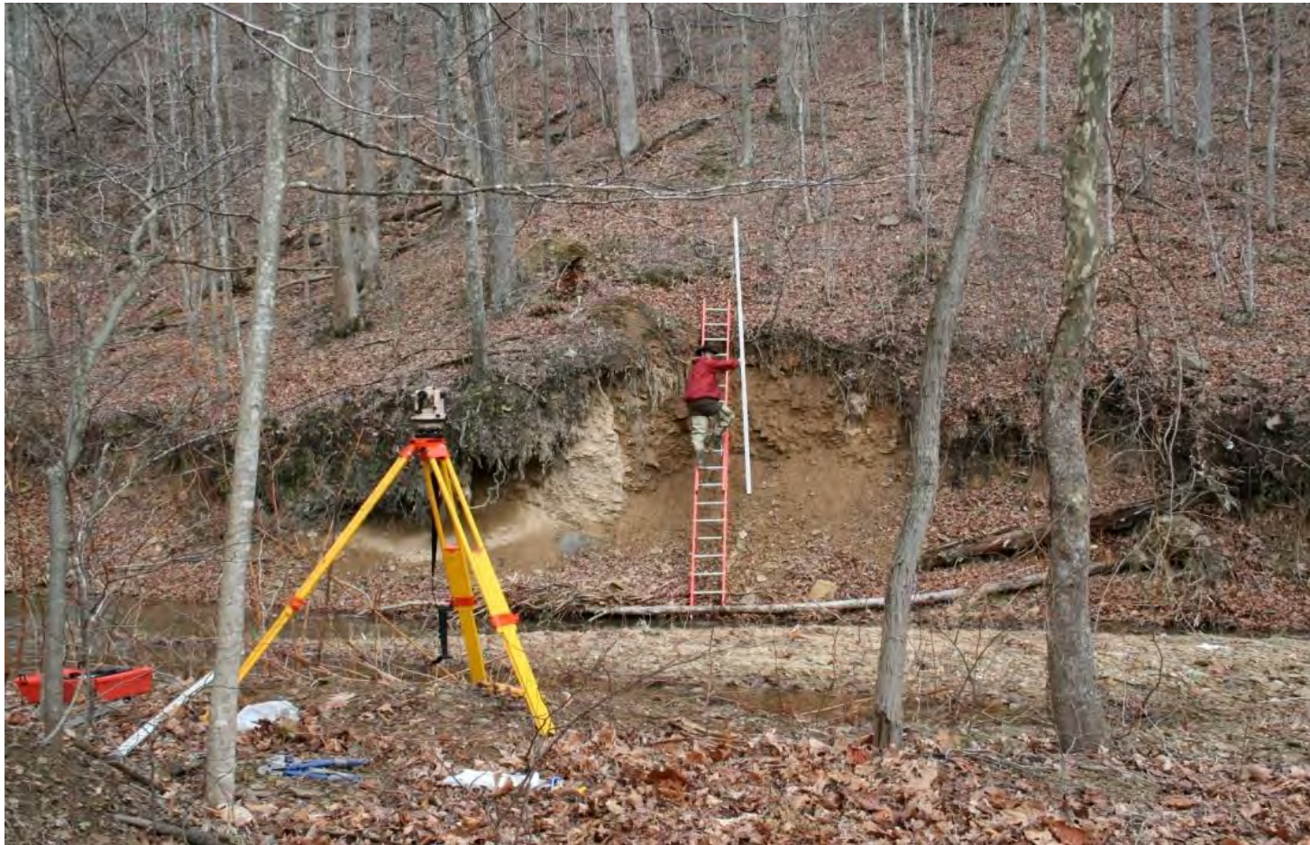
Figure 3.54. Measurement of channel cross-section between fixed end points (4 ft rebar monument pins).
