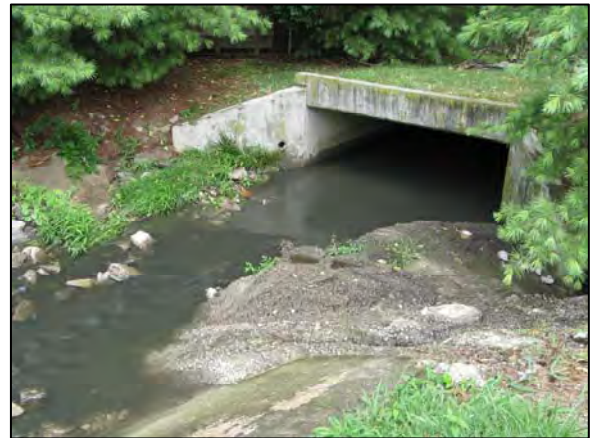
Grey Colored Stormwater on Vaughn's Branch Upstream of Picadome Golf Course
