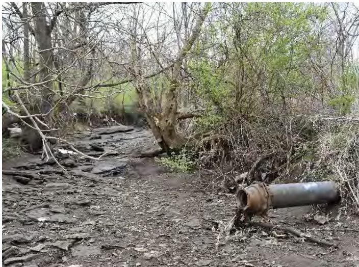
CR5- Bedrock-Drainpipe-Undercut Banks
