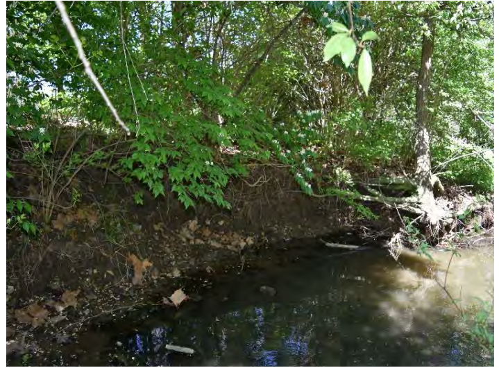
DI- Erosion and Undercut Banks
