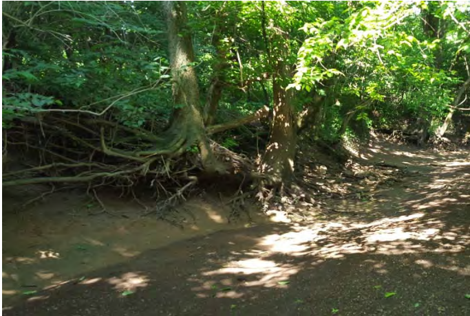
ES-6, Erosion of banks and heavy siltation
