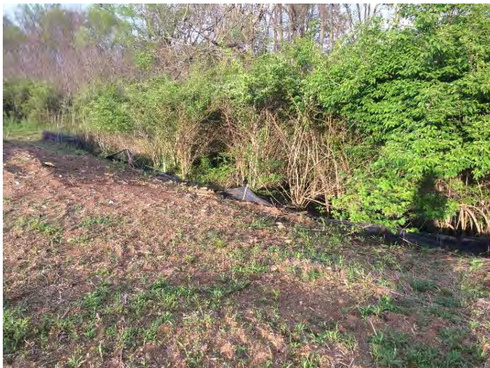
A2- Failed Silt Fence on Lb near Reach
