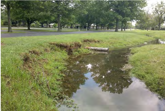
ES-7, Erosion of bank leaves extended pipe in stream
