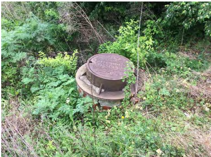
CR9- Sanitary Sewer Adjacent to Stream
