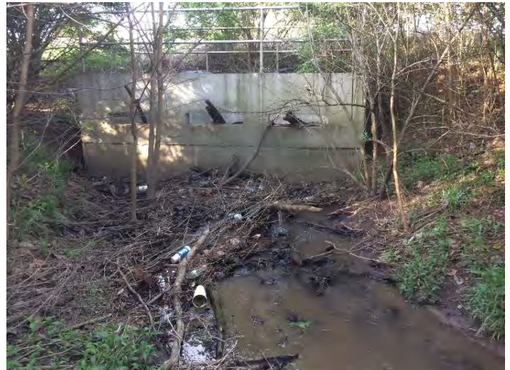
A2- Culvert Filter Facing Downstream, Leaf Packs
