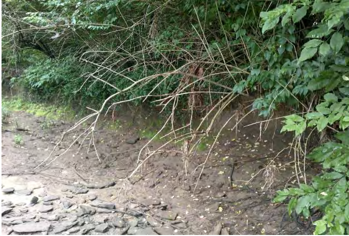
ES-1, Erosion upstream of infrastructure
