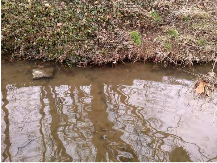
CR6- Under Cut Bank
