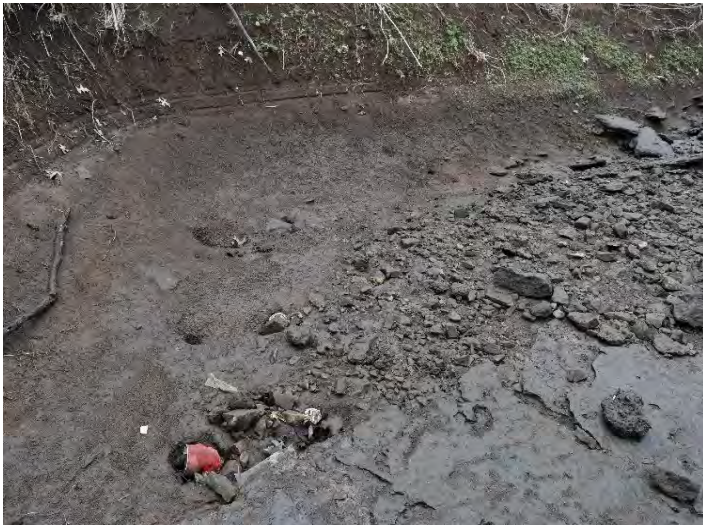
CR5- Drain Holes Bank Erosion
