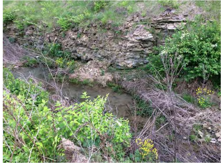
AI- Bank Undercuts 2 (Rb)
