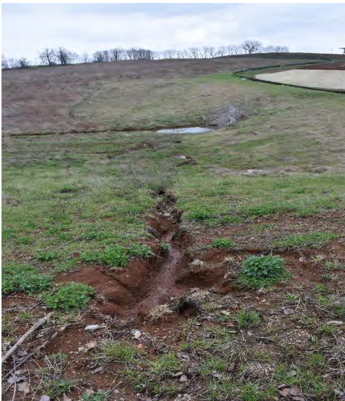
CI- Erosion Entering Top of Reach
