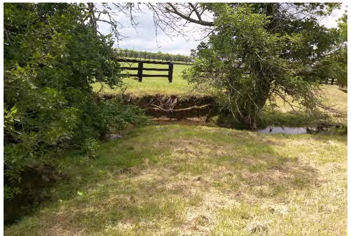
ES-7, Erosion in a bend
