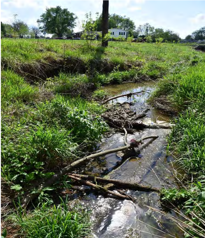
HI - Bank erosion
