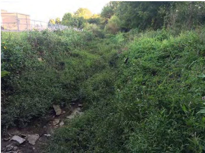
CRI - Pump Station Stream Reach
