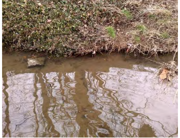
CR-8 UNDER CUT BANK
