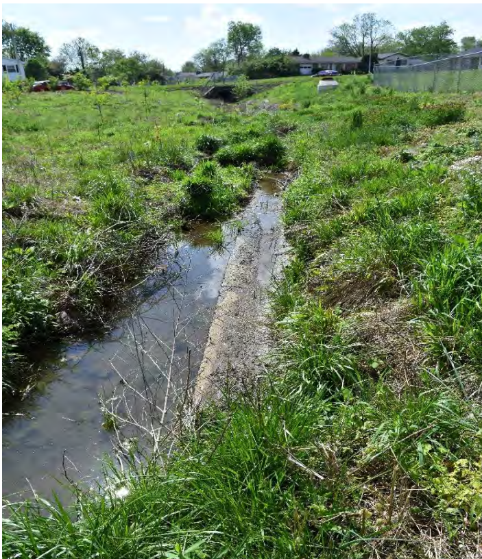
HI- Possible Channelization-Sanitary Sewer
