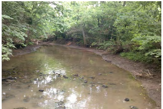
ES-3, Erosion along both banks near road crossing
