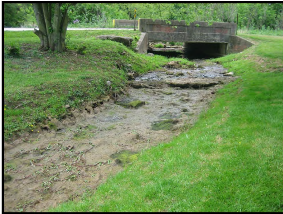
Figure 40. Dry Conditions at Site 9
