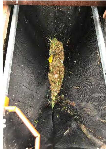
Figure 5.4 Catch Basin Insert Removes Debris Underneath an Inlet
