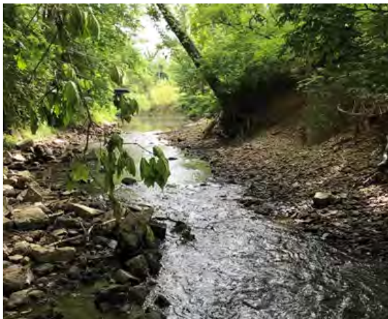
Figure 4.5 Looking upstream: Inner berm erosion and undermining tree root mass
