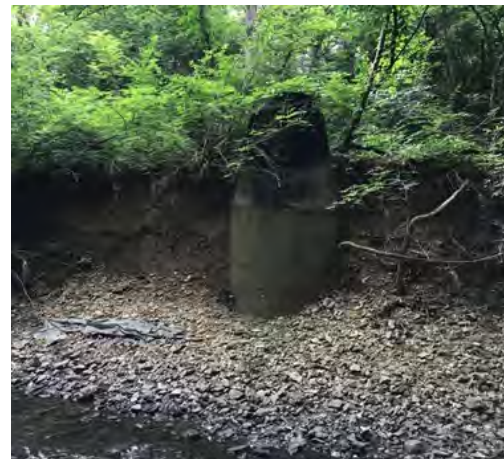
Figure 4.6 Left bank: Vertical stream banks and lateral stream bank erosion
