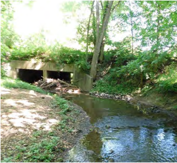
Figure 4.24 Looking downstream: debris jam upstream of Foxboro Road
