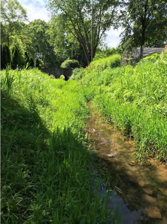
Figure 4.13 Looking downstream: lack of riparian corridor and tree canopy cover
