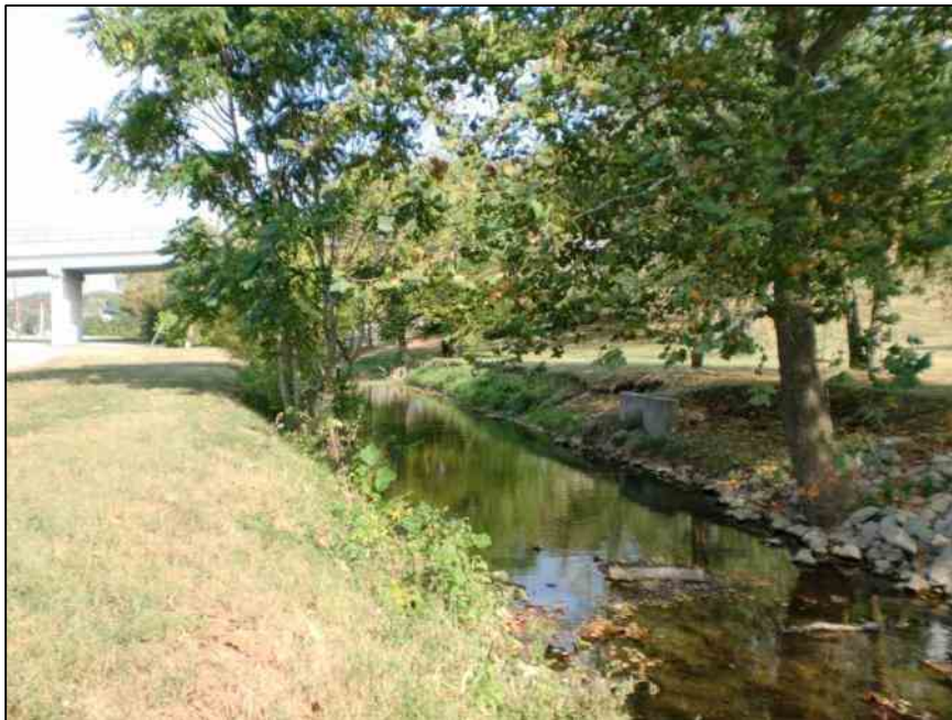
Figure 2-30. Mainstem of Hinkston Creek located in downtown Mount Sterling, west of KY 11 and south of West Locust Street. Note: very little riparian cover and poor bank conditions. (Photo taken by Greg Sousa, Tetra Tech, September 22, 2010)
